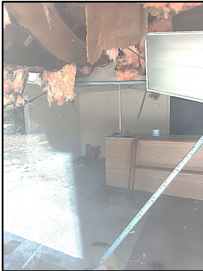
Interior view from a window of the building showing its poor interior condition.
