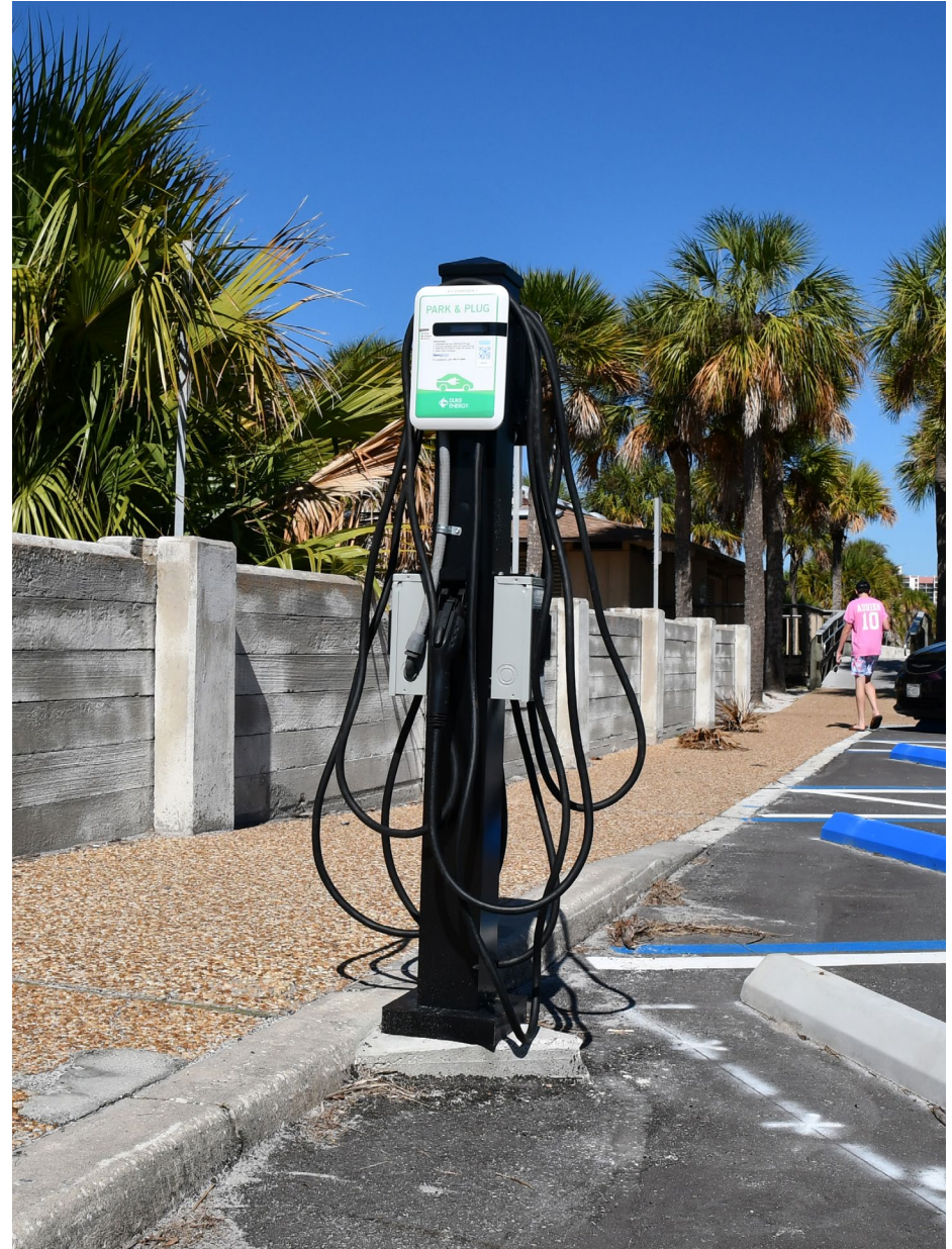
EV charging station at Sand Key Park. Photo credit: Pinellas County
