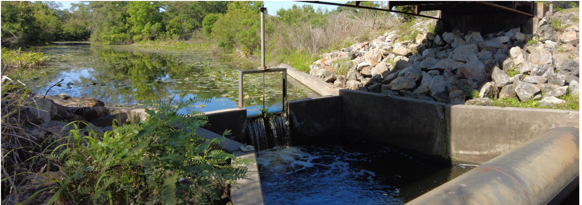
Stormwater management system in Kapok Park
