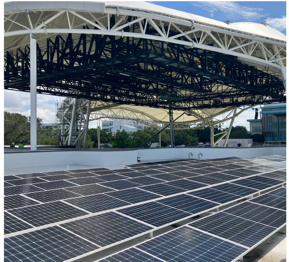
Solar installation on The Sound
