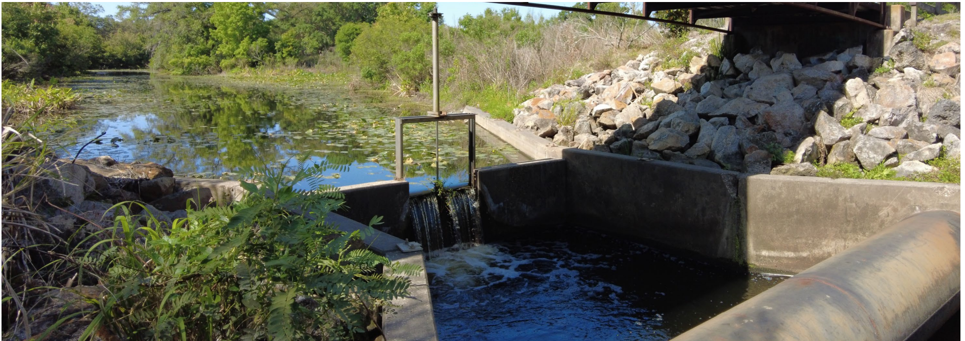
Stormwater management system in Kapok Park
